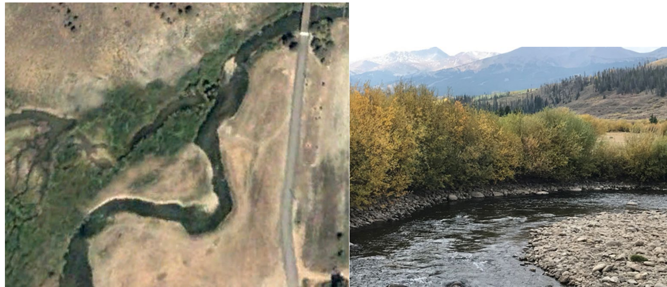
Figure 16. Before (aerial on left) and after picture (on right) of deformable bank construction along the Blue River upstream of Dillon Reservoir in Summit County Colorado
